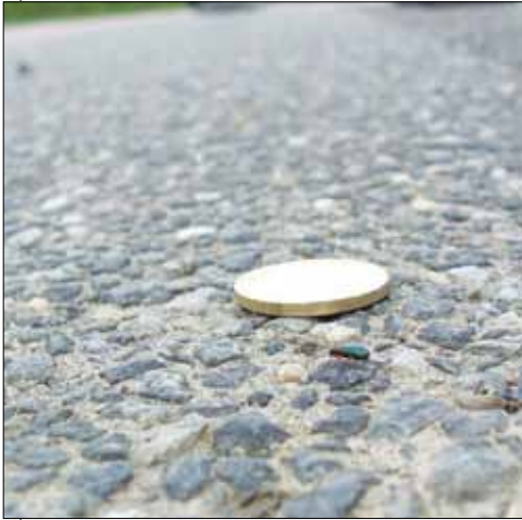
▲ Exposed aggregate surface , seen here on European concrete pavement, may suppress noise while enhancing friction.
