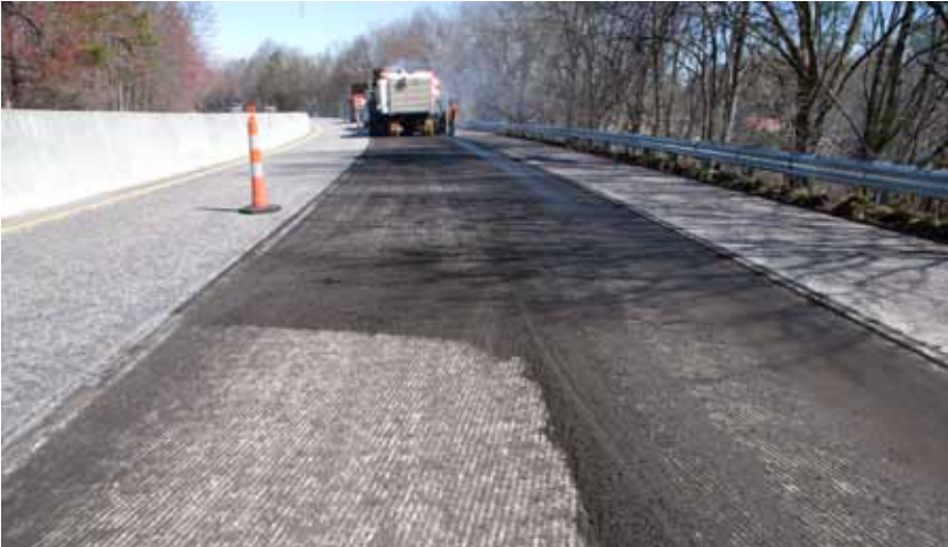
▲ Micromilling, or fine milling, by Pavement Products and Services, provides super-smooth base for overlay while correcting cross-slope problems on I-185 in Greenville, S.C.
