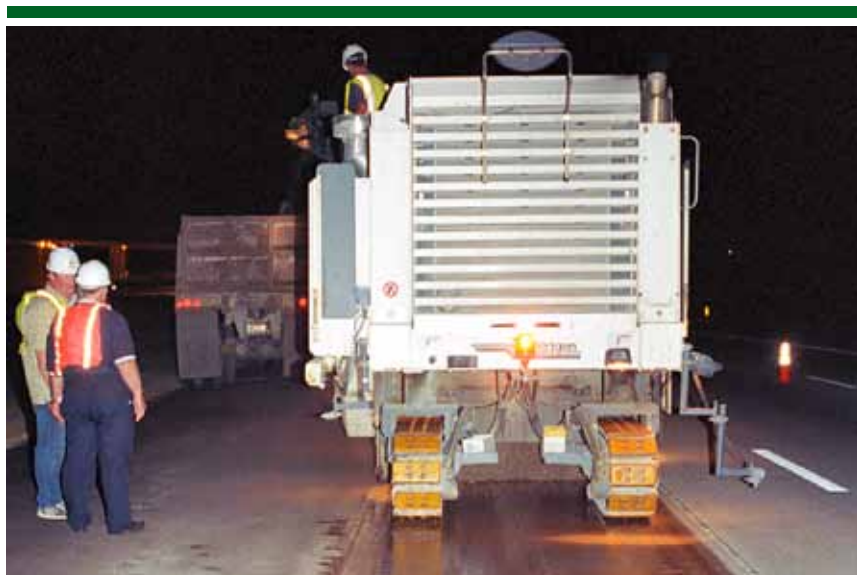
▲ TexOp Construction uses a fine-toothed drum to prep President George Bush Turnpike near DFW Airport in advance of NovaChip overlay; the contractor alternative provided significant savings over diamond grinding originally planned by owner North Texas Tollway Authority. Photo credit: Wirtgen America, Inc.
