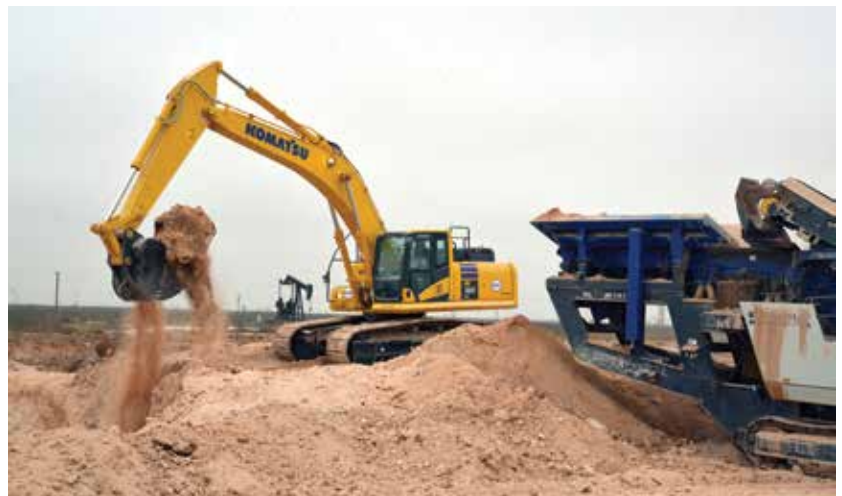
Oil extraction and well service industry drives much of demand for crushed aggregate; at Cooper Pit, Jones Bros.' MR 110 ZS EVO operates in shadow of oil rig
