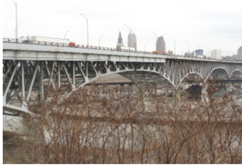
Ohio's Innerbelt Bridge carries I-90 over the Cuyahoga River just south of downtown Cleveland.
