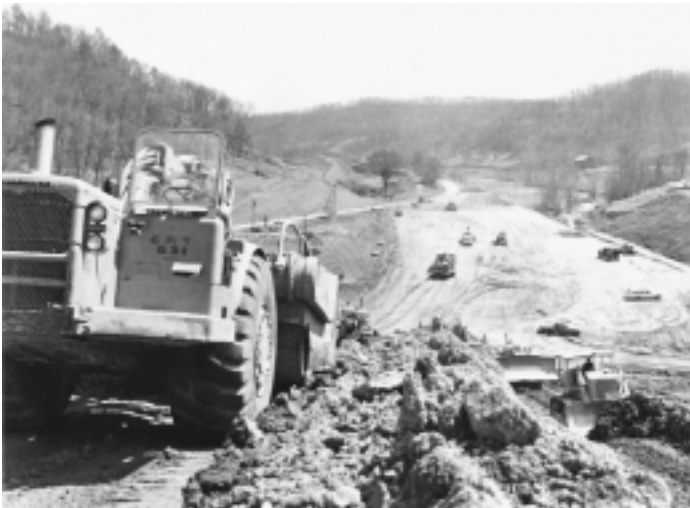
Top: The I-70 westbound viaduct over the Kansas River between Kansas City, Mo., and Kansas City, Kan., nears completion in November 1962. Above: I-64 is constructed west of Grayson, Carter County, Ky., in 1967.
