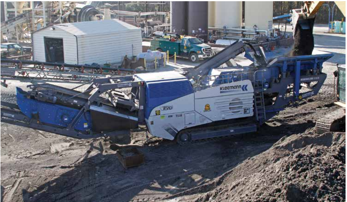
TOP: For C.W. Matthews, the Mobirex crusher is fed by an excavator rather than a front end loader. Fines off prescreen (center) bypass the crushing circuit and are conveyed to a super stacker where they rejoin half-inch minus material. BOTTOM : The two Mobirex impact crushers are moved around among 26 asphalt plants throughout the company. "The hopper wings fold hydraulically, there are no tools involved," Greg Taylor said. "The only thing we really must do is take the side discharge belt from the prescreen off."
