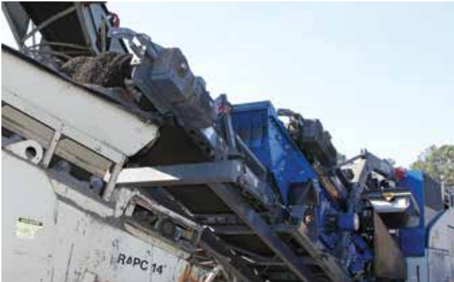
TOP: At the C.W. Matthews Forest Park, Georgia, plant are general superintendent Greg Taylor and crushing foreman Johnny Jones. BOTTOM: The conveyor-mounted screen eliminates the need for a stand-alone screen, contributing to a compact footprint that lets the impactor sit within the hot-mix plant layout.
