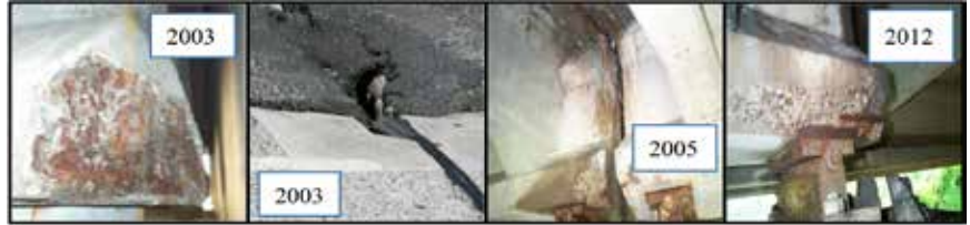
Progression of deterioration of precast girder, New Jersey. PHOTOS: Lou, Nassif, Su and Truban
