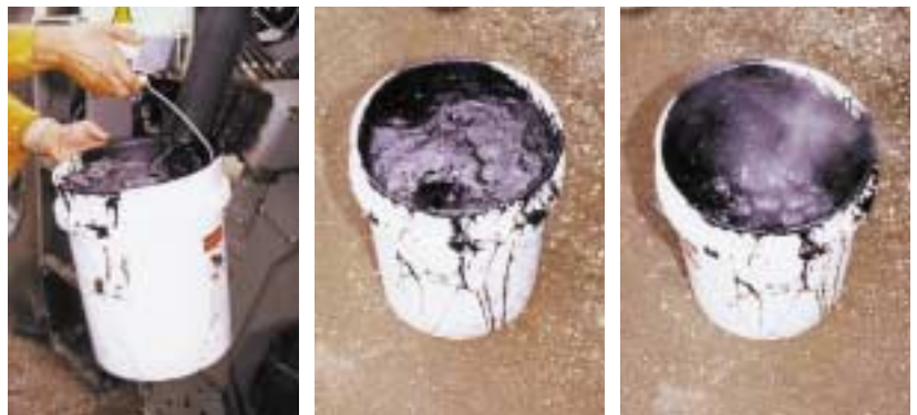
Sample of foamed asphalt is drawn from WR 2500, foams to many times its volume, and subsides within seconds; millions of bubbles act as carrier of liquid asphalt cement to road base fines in Wirtgen WR 2500 road recycler
