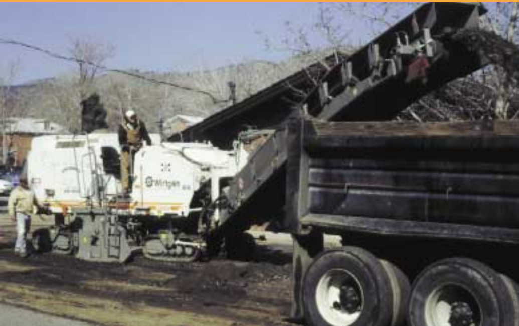
W 1900 DC works in constrained quarters of parking lot in historic downtown Golden
