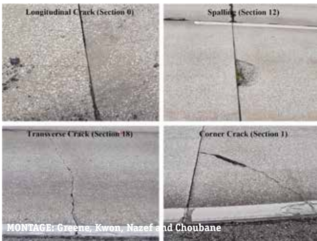
Distresses observed in the Florida overlay test sections.
