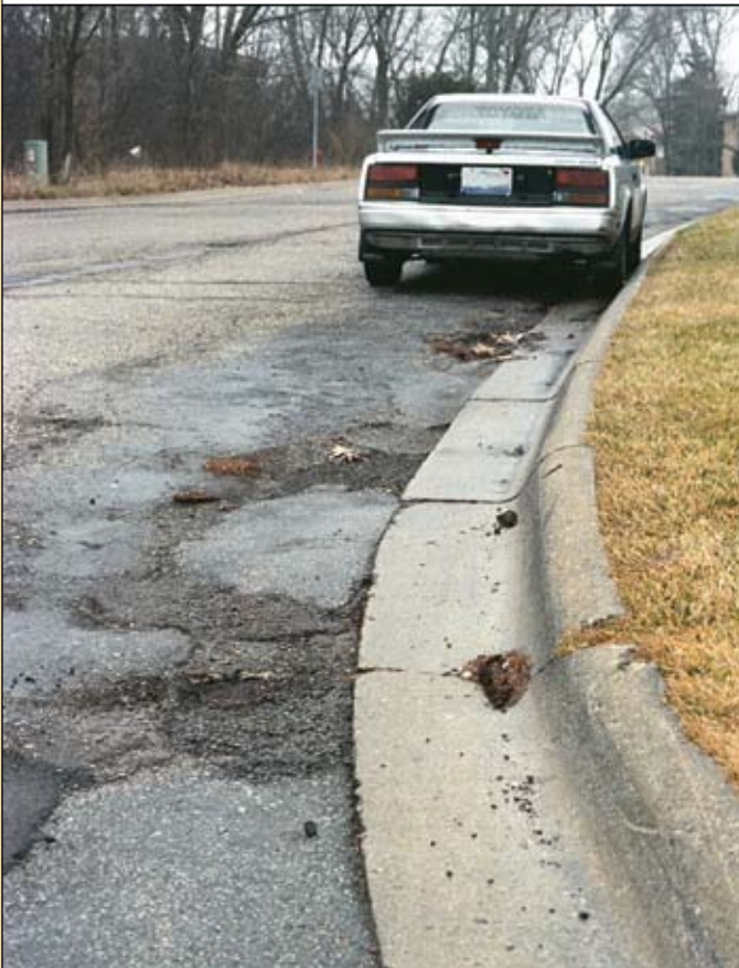
▲ Structural cracking and potholes must be repaired before surface treatments are placed.
