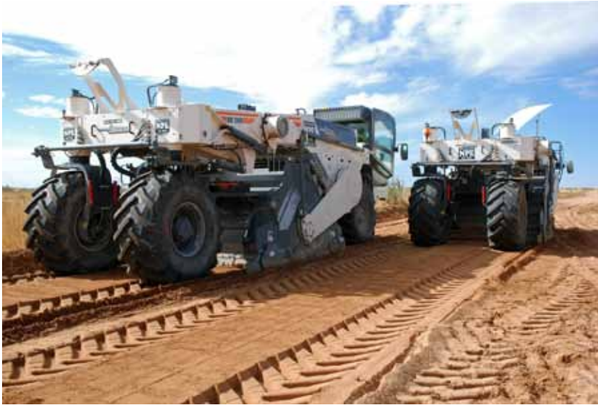
▲ For new alignments, stabilize subgrade prior to work on subbase, base and pavement layers.
