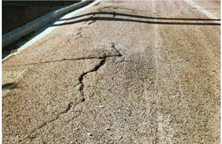
▲ If not stabilized, expansive subbase and base layers will heave and destroy pavement.
