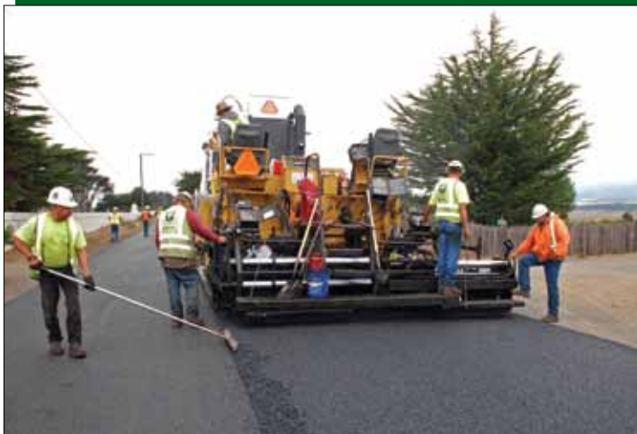
▲ On California's Pacific Coast Highway 1 , warm-mix asphalt is placed with minimal emissions near town of Point Arena.
