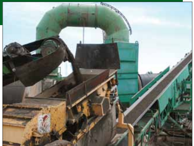
▲ In Minnesota , crushed and screened reclaimed asphalt pavement (RAP) is fed into a plant to provide lower-carbon footprint paving.
