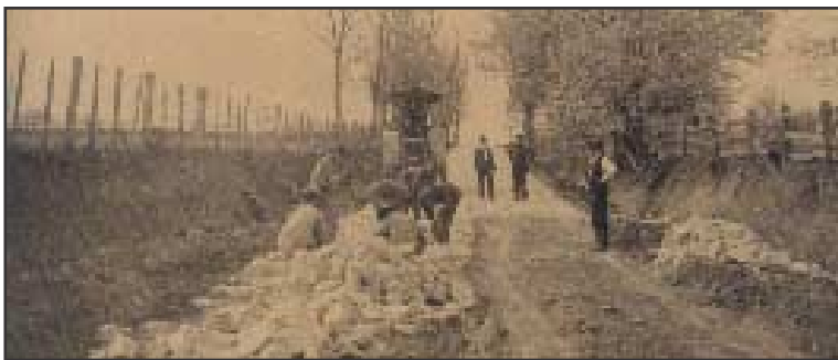
Workers break up stone by hand at this road construction site in Luzerne County, Pa.
