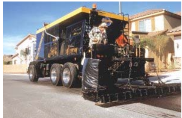
Slurry machine operator plays critical role in ensuring slurry mix is being applied correctly
