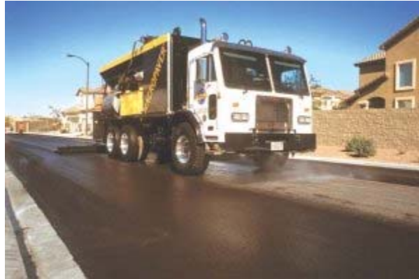
Dedicated slurry surfacing truck applies slurry to residential street in suburban Las Vegas, Nev.
