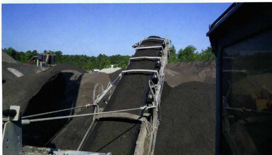
The cold central plant recycles RAP into foamed asphalt at full capacity for owner Allan Myers for use on the I-64 project.
