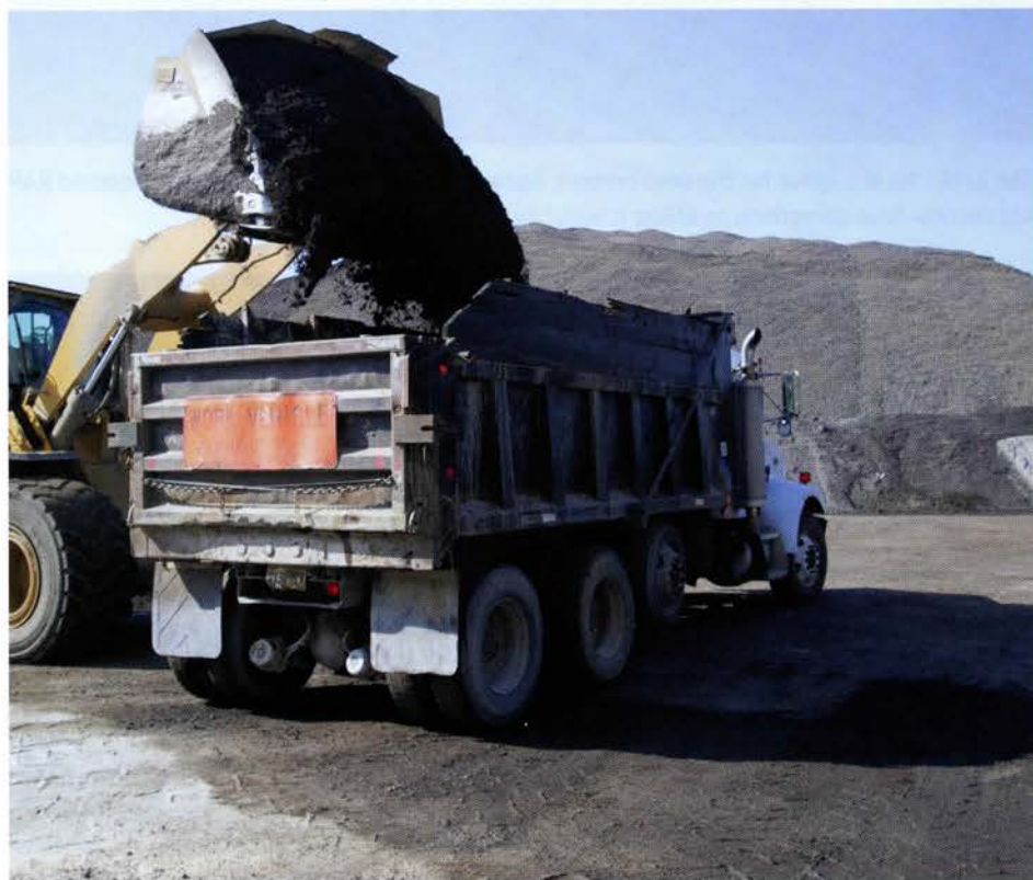
They start making foamed asphalt base mix early in the morning, prepping it to ship out to I-64.
