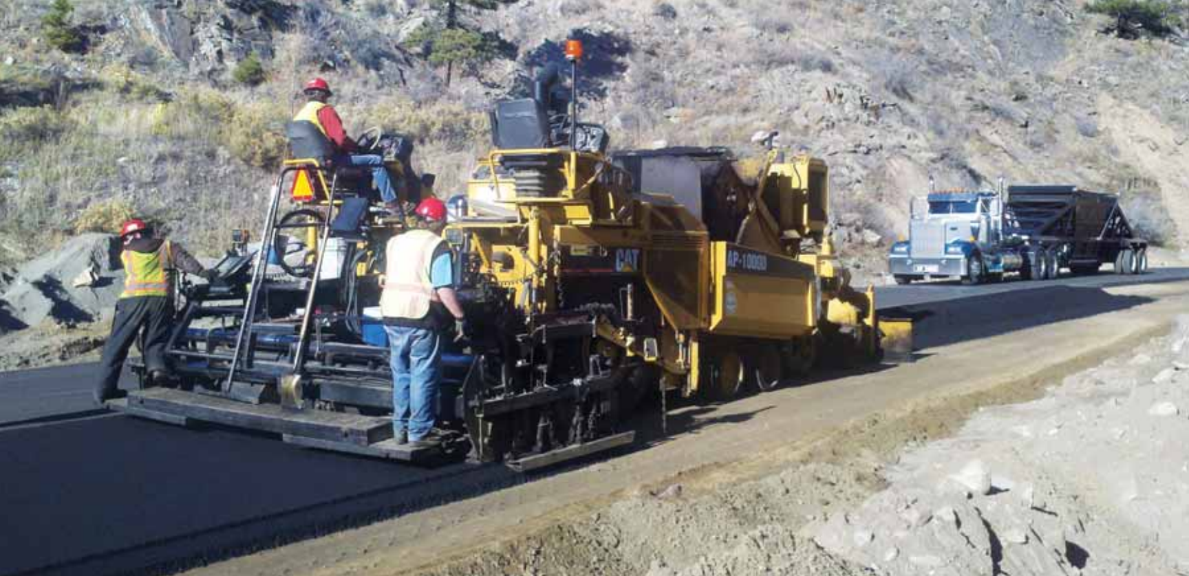
To maintain asphalt workability, forces of Coulson Excavating pave U.S. 34 between Loveland and Estes Park with warm-mix asphalt due to long hauls of up to three hours, low ambient temperatures at the end of the season and high elevations. Photo courtesy of MWV Evotherm.
