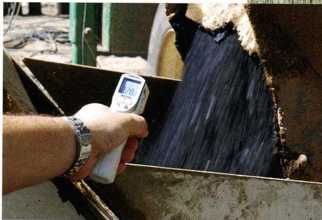
At plant, warm mix ranges from 225 to 235 deg F, compared to 280 deg F or more for conventional hot mix asphalt.
