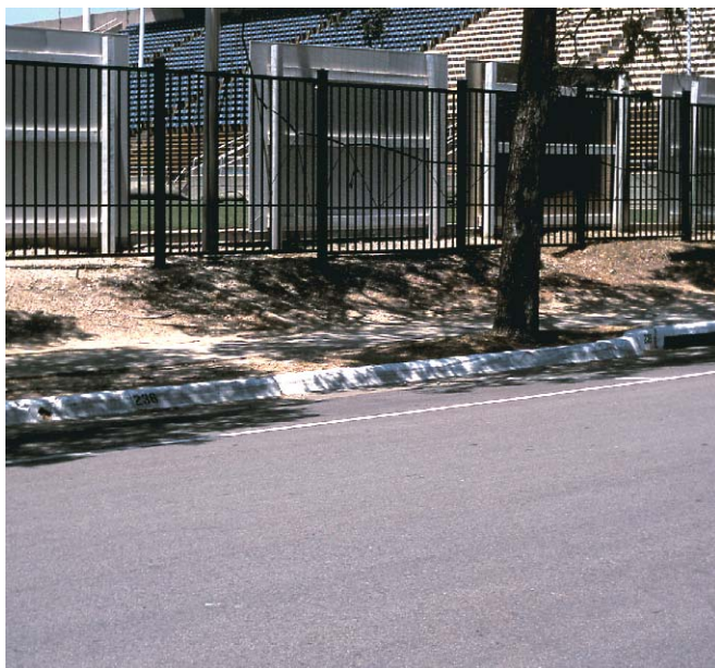
Westchester Drive at Highland Park High School, University Park, Texas, was HIP recycled in 2003.
