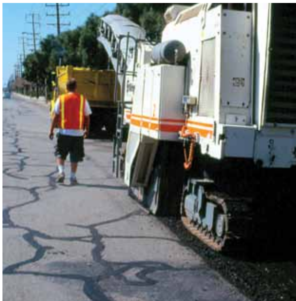
▲ When random cracks get to be too much, it may be time to renovate pavement with a mill-and-overlay.
