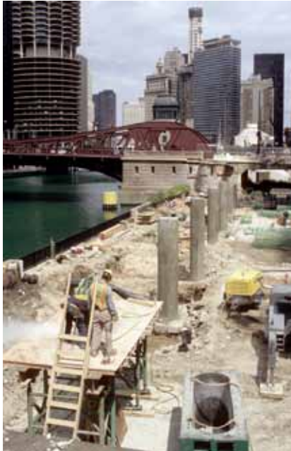
▲ Quaternary concrete mix is used for Revive Wacker Drive project for City of Chicago.
