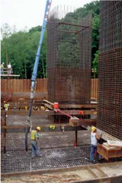
▲ GGBF slag cement – in a 70 percent substitution for Type II portland cement – is being used to lower the heat of hydration in a 2,600-cubic yard mass pour for a pier footing for the Phase 1 extension of Page Avenue in St. Louis County.
