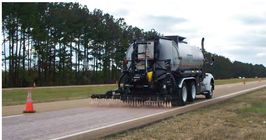
Asphalt rejuvenator is placed on U.S. 25 near Jackson, Miss., using a BearCat 2,000-gallon distributor on an abraded surface.
