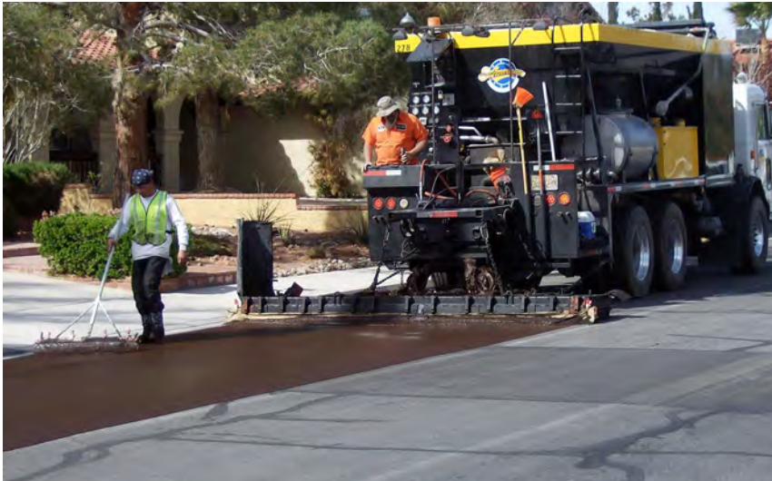
Unit of American Asphalt and Grading Company places slurry seal as part of year-long work with the City of Las Vegas in 2009
