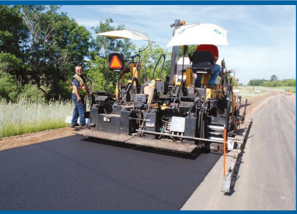
In Crow Wing County, Minn., warm mix asphalt containing Evotherm additive is placed in effort to minimize low-temperature thermal cracking while avoiding costly high-performance PG asphalt binder.
