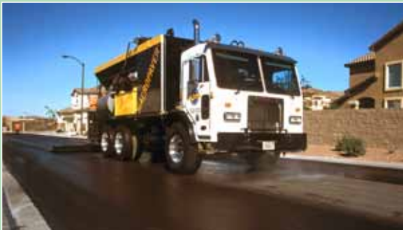
▲ Slurry surfacing is a step beyond conventional chip seals and requires specialized application equipment, but with potential benefits. Photo courtesy of VSS Macropaver
