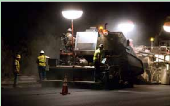
▲ A rubberized thin wearing course is placed by Sunland Asphalt on California State Highway 99 south of Fresno; high-performance surface treatment prolongs highway's life while standing up to brutal California traffic. Photo courtesy of Vögele America
