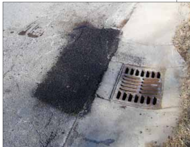
▲ As illustrated in these pictures (from top to bottom) existing damaged pavement; repair is squared, cleaned of debris and tacked; final repaired pothole.
