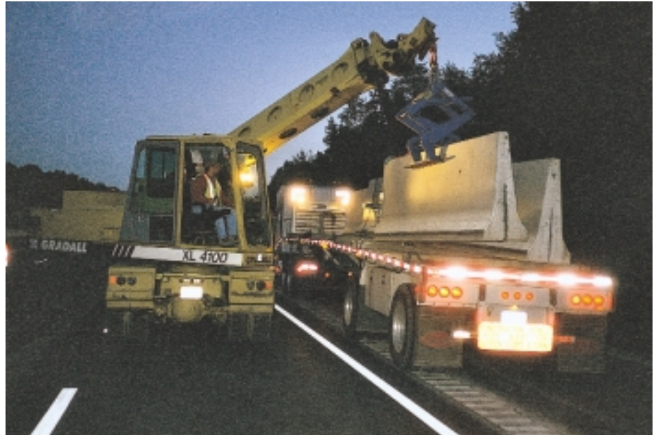
Given the incredible traffic volumes on our Interstate system, night work has become a fact of life in the post-Interstate era. Here, jersey barriers are placed ahead of night work under traffic in Pennsylvania.
