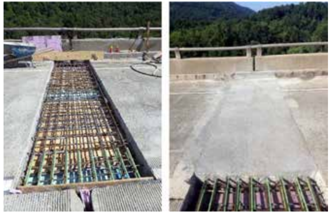
In the Virginia I-64 bridge experiment, researchers studied high-performance fiber reinforced concrete pours over pier caps. IMAGES: Ozyildirim, Khakimova, Nair and Moruza.
