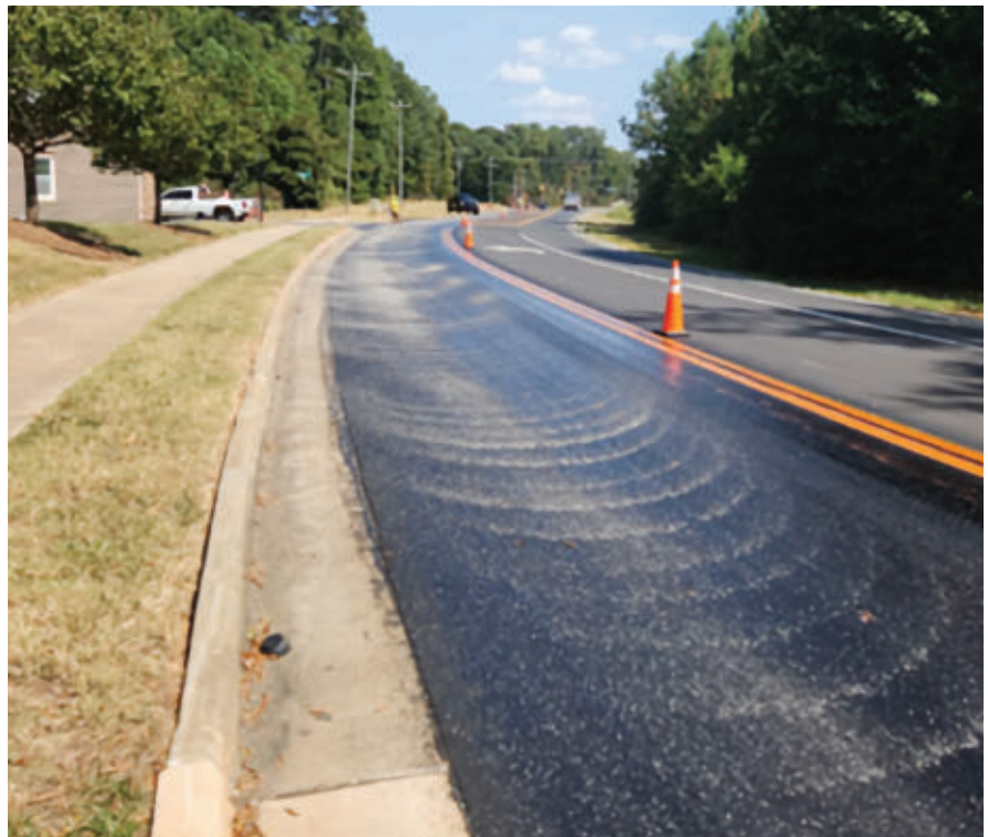
In the Tarheel State, a light application of fine aggregate is applied immediately after treatment
