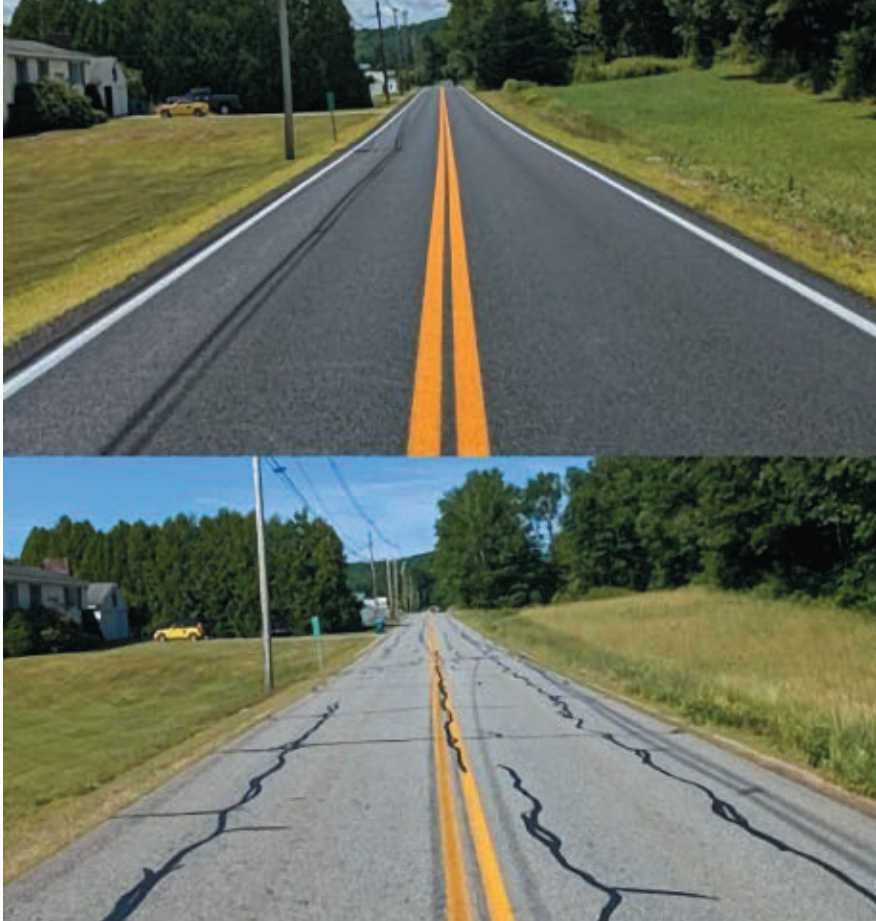
On Mass. Route 32 in Hardwick, preserved pavement with asphalt rubberized chip seal as-built (above) and pre-application (below)
