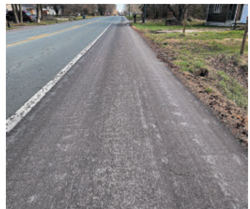
As-built Delaware shoulder rut after micro placement, March 2026
